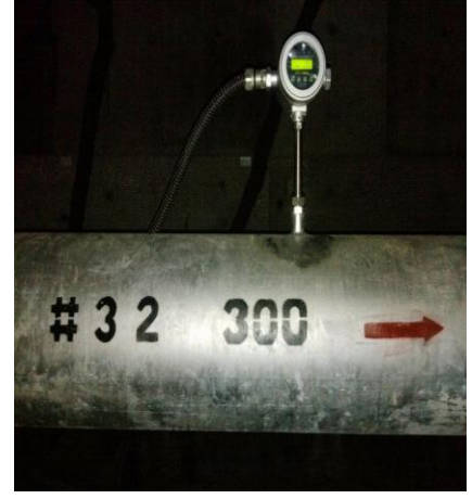
Tancheon Environment Co., Ltd. Delivery of 196 units for measuring air flow in the aeration tank
