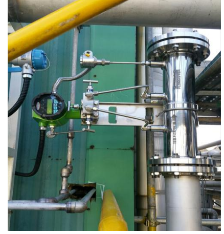
Hanwha Ulsan Plant Air, 100A Line
