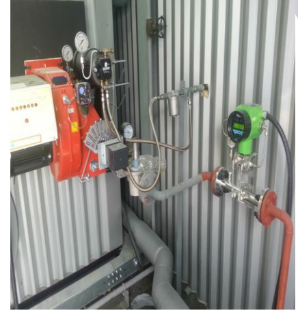
Icheon (Residual Body Disposal System) LPG, 25A line
