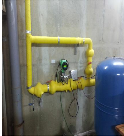
City Railway Corporation Water, 50A Line
