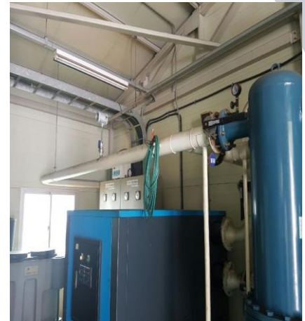
Delivered 203 units for compressed air to Daegu Dalseong Industrial Complex Energy
