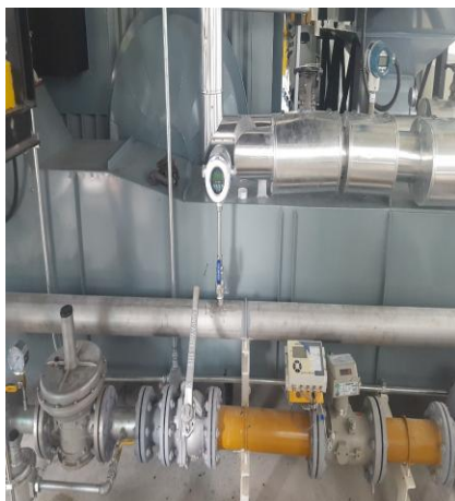
Gwangju Environment Corporation Biogas, 100A line
